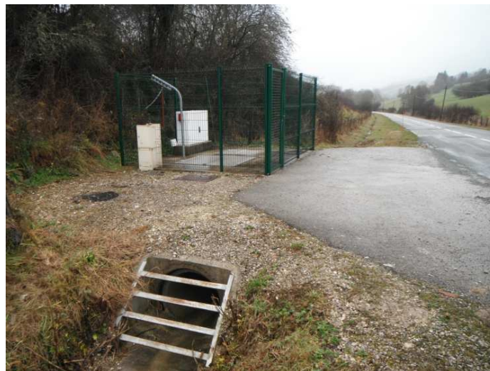
Station de relevage de Fuans.
